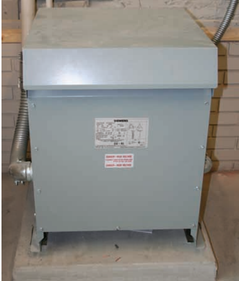
Transformer (Consumer Owned) Dry Type
