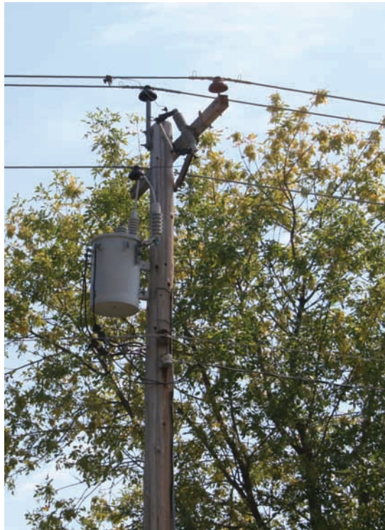
Transformer (Utility Owned-Pole Mounted) Oil Filled
