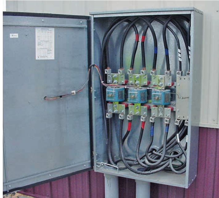
Current Transformers inside the Cabinet
