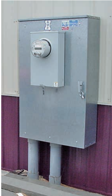
CT Cabinet and Meter Socket
