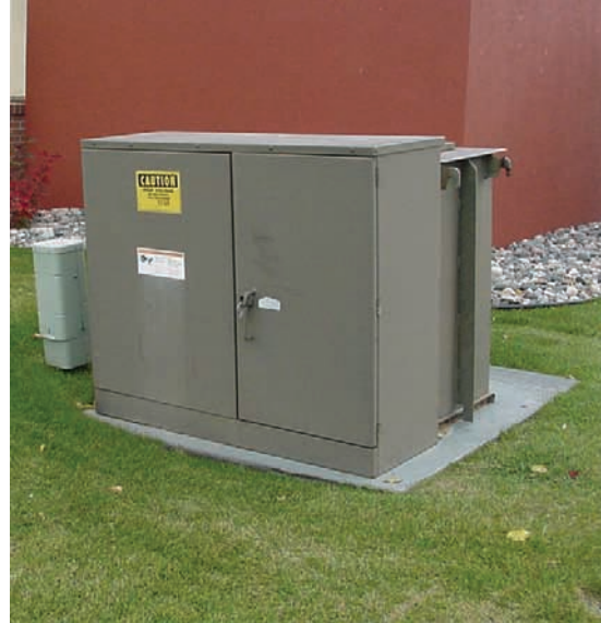
Transformer (Utility Owned-Pad Mounted) Oil Filled
